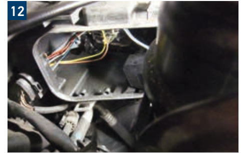
12 → There is now enough space for the bulb to be replaced.
